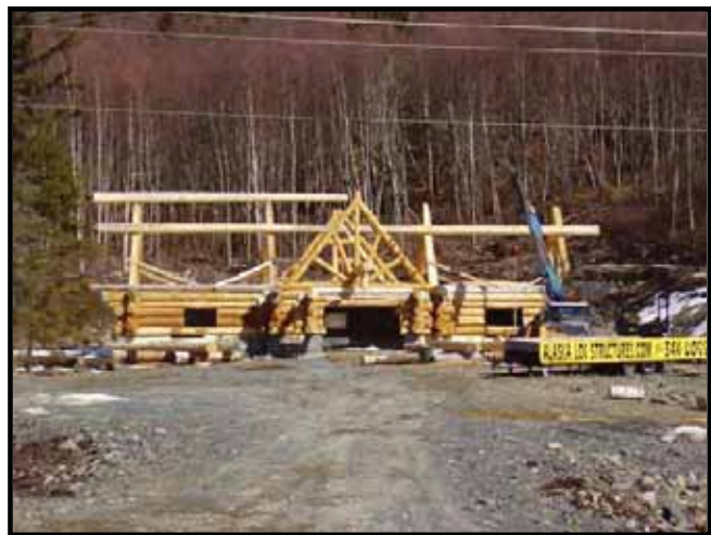
Photograph 32 – Log structure being developed north of the Seward Highway at approximately MP 99.5.
