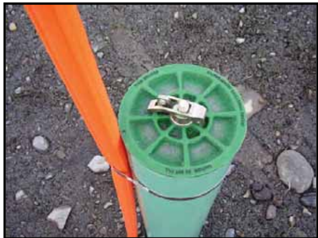
Photograph 9 – Essential Gas Station leach field vent pipe.
