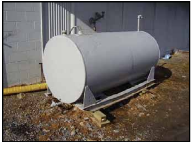
Photograph 5 – Essential Gas Station heating oil tank.
