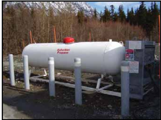
Photograph 7 – Essential Gas Station propane storage tank.
