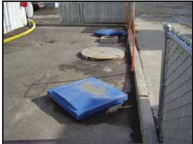
Photograph 2 – Essential Gas Station gasoline USTs.
