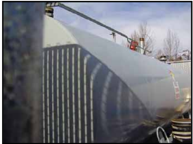
Photograph 6 – Essential Gas Station 10,000-gallon aboveground diesel tank.
